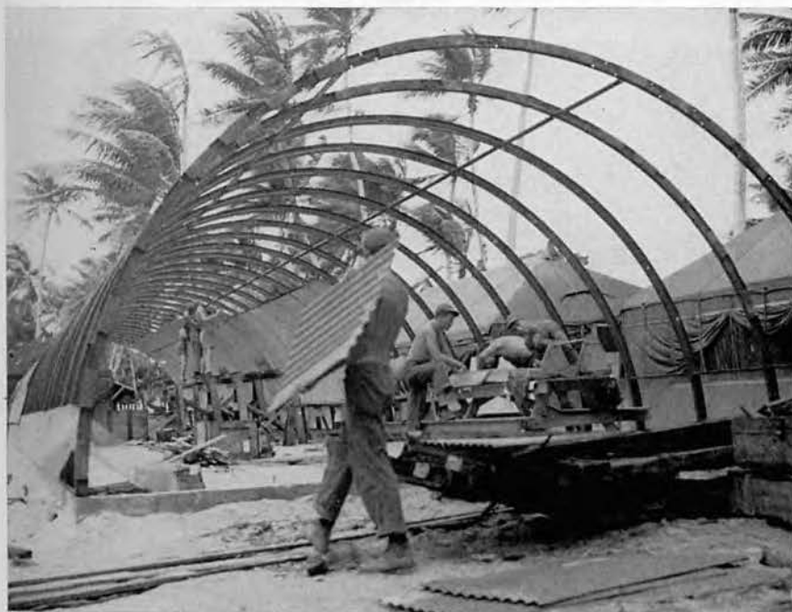
No time to waste, the deck, the sides, and the bulkheads are done in one operation.
