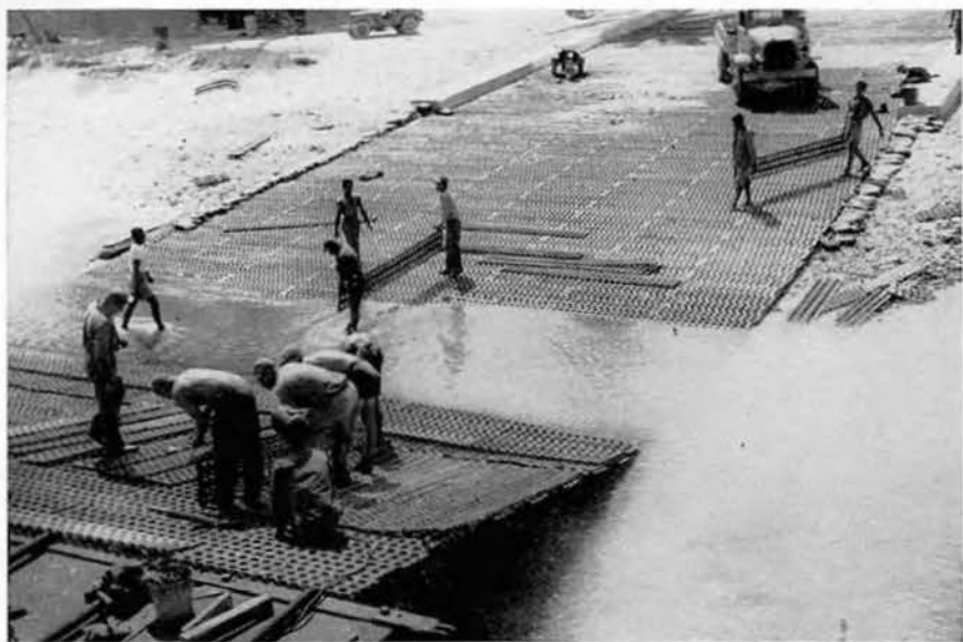
The layers of steel matting insure flexibility, as the ramp nears completion.
