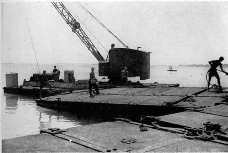
These water filled and rusty pontoons are repaired by the barge crew and welders, before the dock is assembled.
