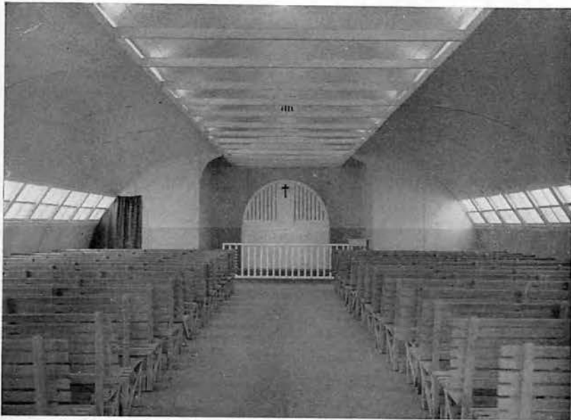
Masters of their trade, the painters and electricians turn a quonset hut into a beautiful edifice.
