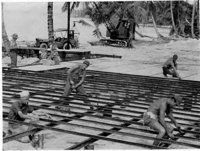
On leveled area, floor joists are set on coconut logs, followed by the plywood deck.
