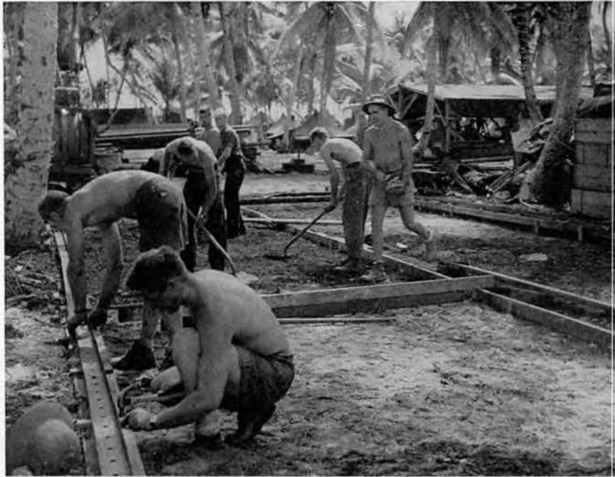
Setting the forms for a concrete deck is the beginning of a quonset hut.
