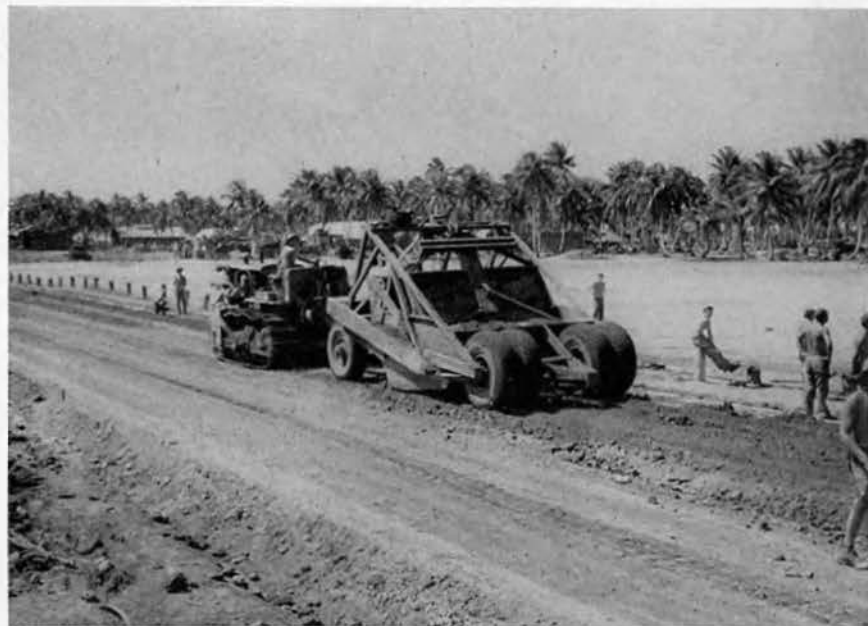
Filling the low spots kept the road free of water, even in the heaviest storms.
