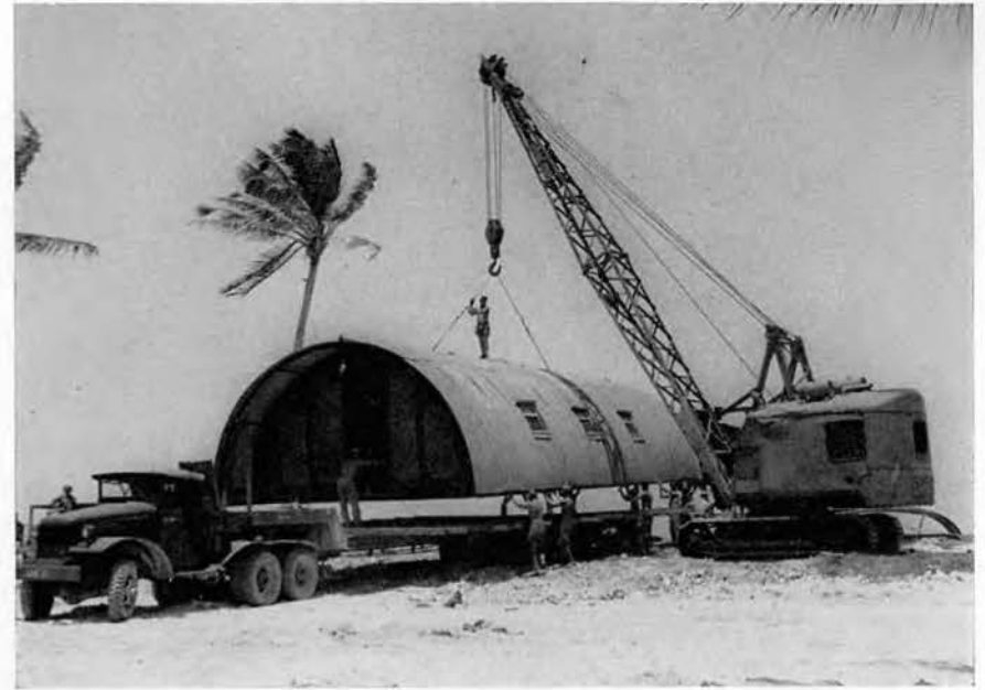
The crane hooks on and is ready to place the hut on its new foundation.
